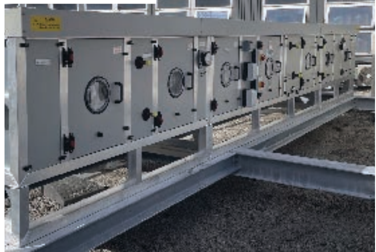
AHU Isolation Units
