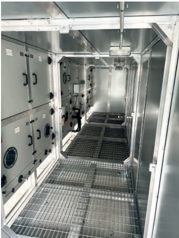
AHU with Maintenance Corridor
